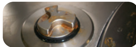
Contaminated iron filings on equipment – the ideal scenario for serious corrosion problems to occur.
