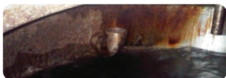
Water supply reservoir with noticeable corrosion; possibly due to the evaporation of hypochlorite.
