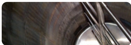
Corrosion of a tank; possibly caused by continuous use (no air self-passivation) or poor choice of products.
